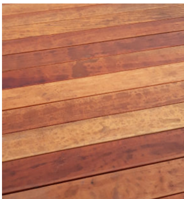
Stains due to excessive oil application
